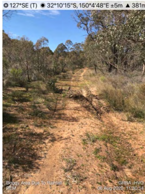
Figure 109 - Boggy area identified on a track within the HVO portion of the Goulburn River BA.
